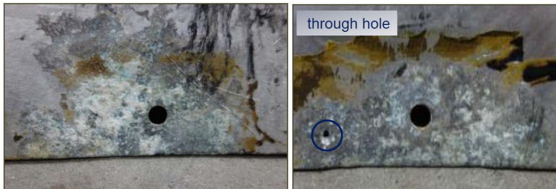
Figure 15: Expanded view of corrosion around fastener holes.
